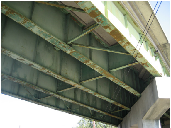
The I-16 Exit Ramp spur completed in the 1960's does not allow most surface street connections through the area, and being almost 50 years old, it is showing increasing signs of wear.
